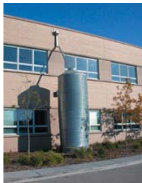
a cistern system collects rainwater from Chicago Center for Green Technology (Chicago, IL) (Photo: Conservation Design Forum)
