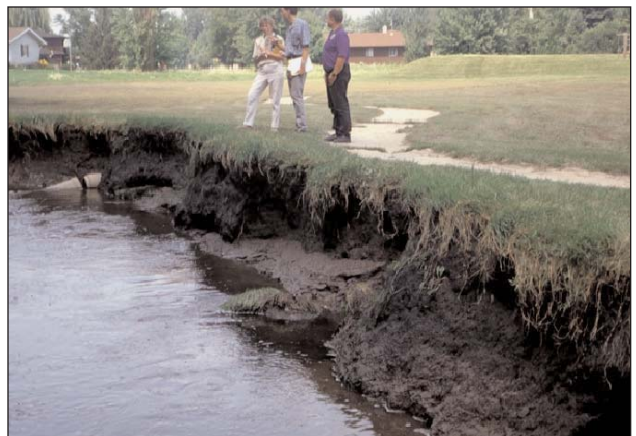
Conventional stream corridor in urban area with significant streambank erosion. (Note exposed storm sewer tiles on left due to bank recession.)
