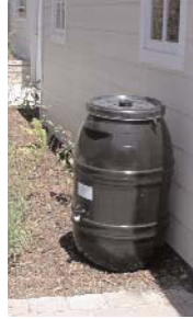
Rain Barrel installed on the side of a residence
